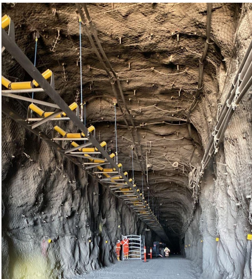
Figure 1: Following completion of the Guajes Tunnel in December 2023, significant progress has been made on the seven-kilometre conveyor with 78% of conveyor tables installed
