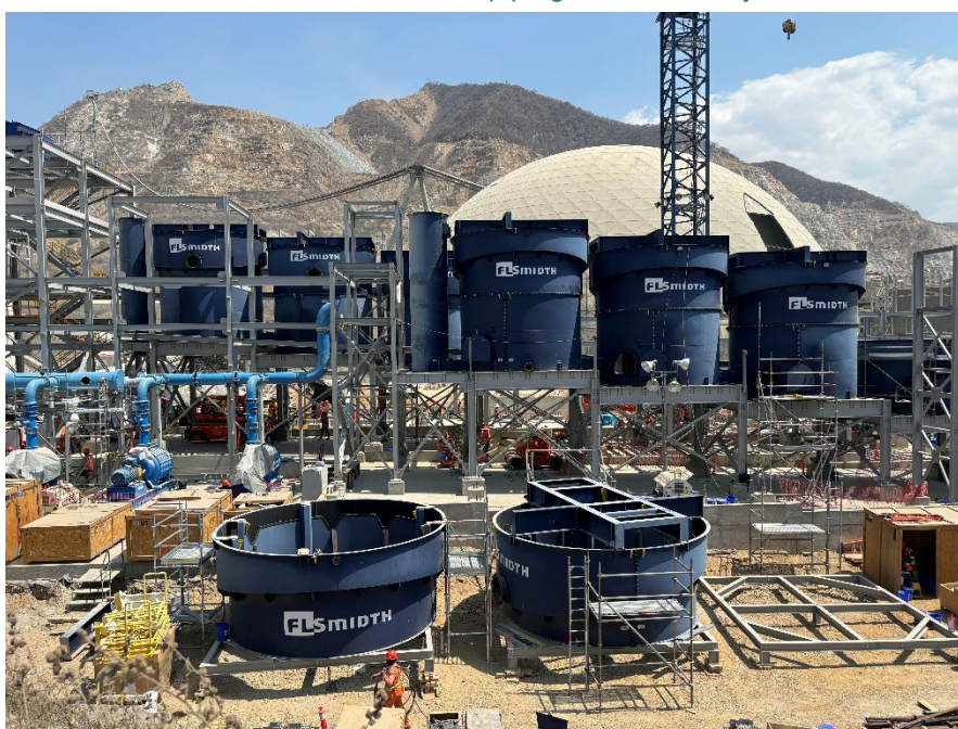
Figure 2: Construction of the flotation facility is progressing well with installation of the copper and iron sulphide flotation circuits and piping well underway
